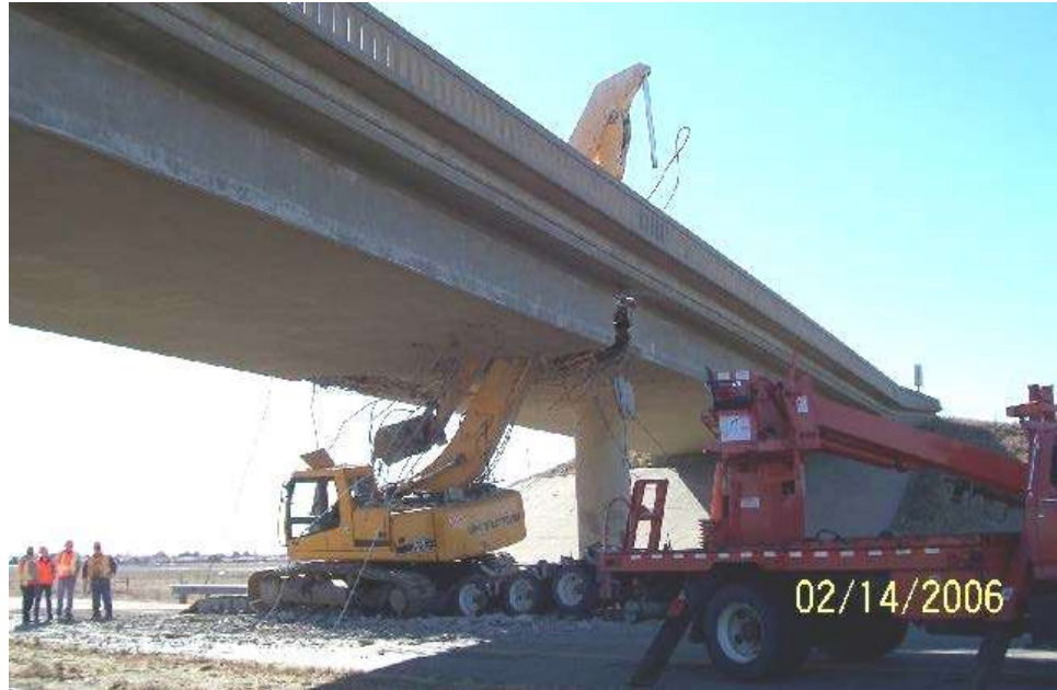
Figure 4.4.2 Accident Involving Construction Equipment and a Bridge
