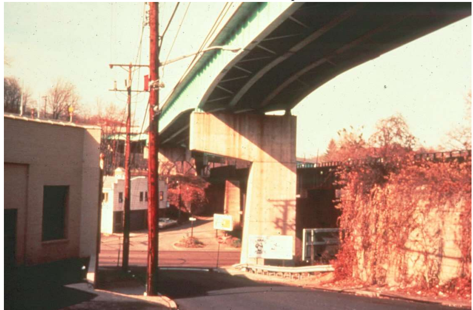
Figure 3.1.6 Unusual Concrete Shapes
